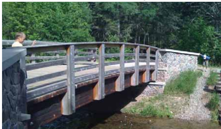
A pedestrian bridge across the headwaters of the Mississippi River in Itasca State Park, MN provides access and views of creek habitat.
