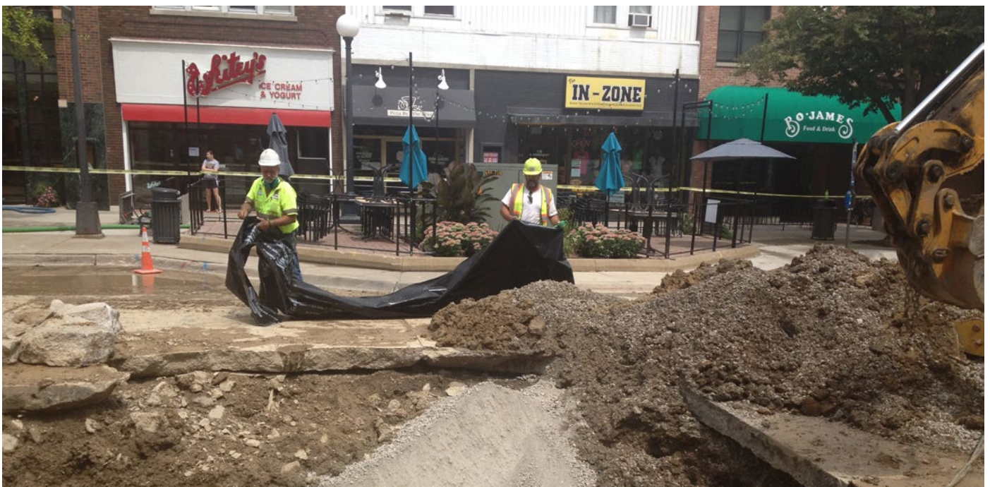
Water main break along Washington in August 2013
