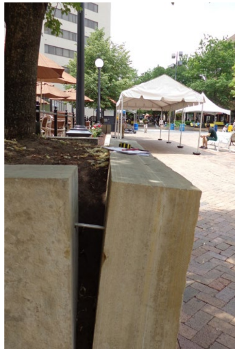
Many of the existing limestone planters are separating and are in need of repair.
