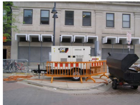
Temporary generators along Iowa Avenue
