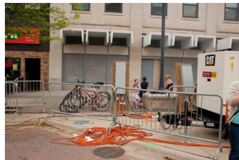
Running power cords during events is problematic
