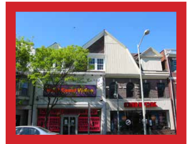
Example of storefront and signage that has significantly modified the building facade and concealed architectural features with inappropriately located signage.
