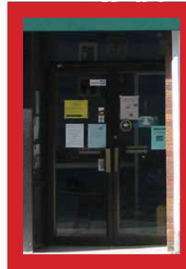
Temporary handbills and other opaque displays should be limited in number and size to keep entries open and inviting.
